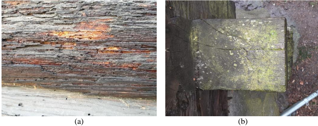
Figure 5: Biological defects in Heierstad Loft
