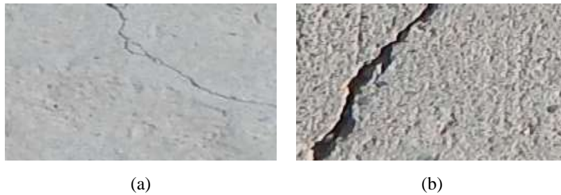
Figure 3: (a) Cracked image with 135° crack orientation (b) Cracked image with 45° crack orientation.
